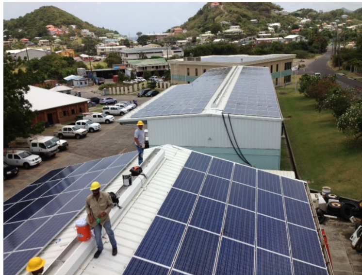
PV at Grenlec
