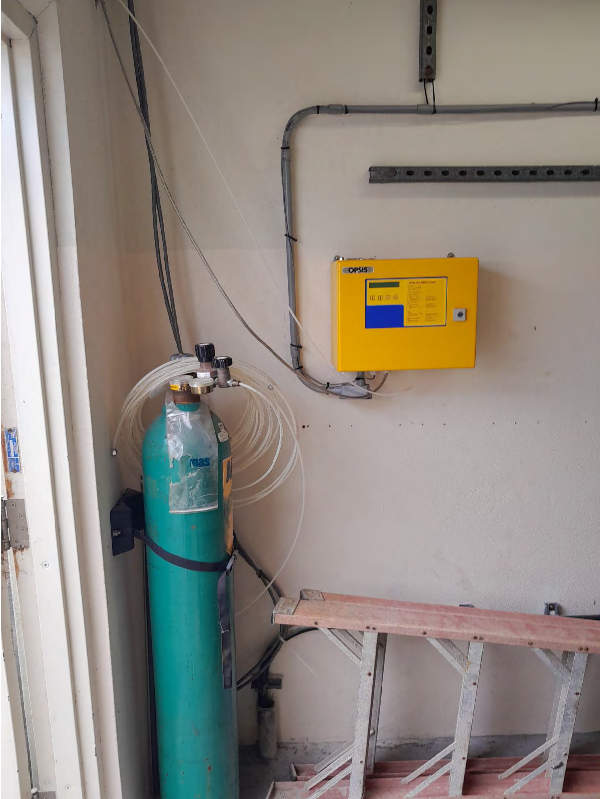
Photo 23 Gas Bottle to be Relocated to Bottle Shed
