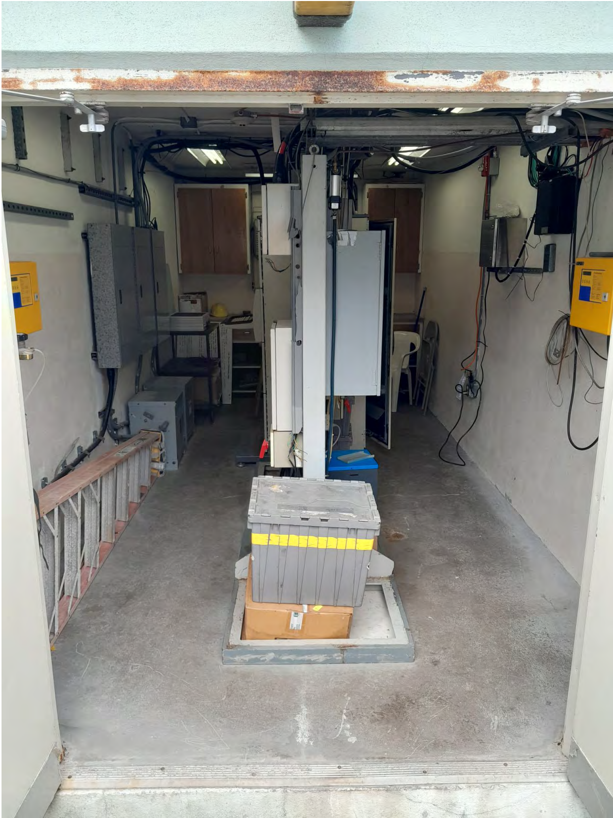
Photo 18 Inside Monitoring Building
