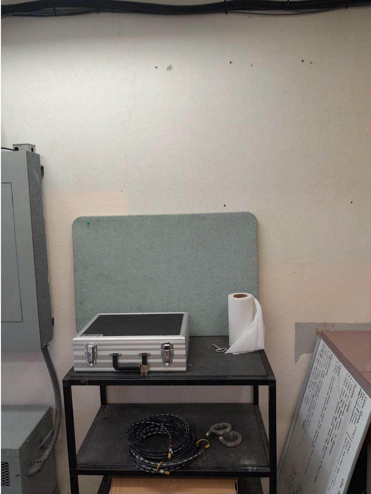
Photo 27 Walls to be Repaired
