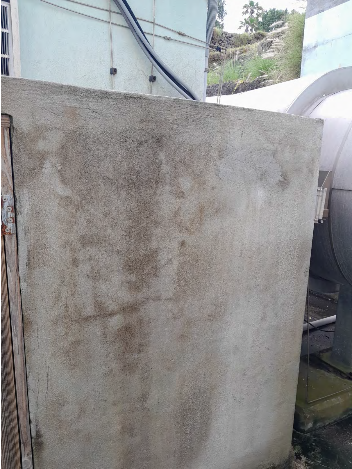
Photo 10 Bottle Shed with CEMS Equipment Enclosed
