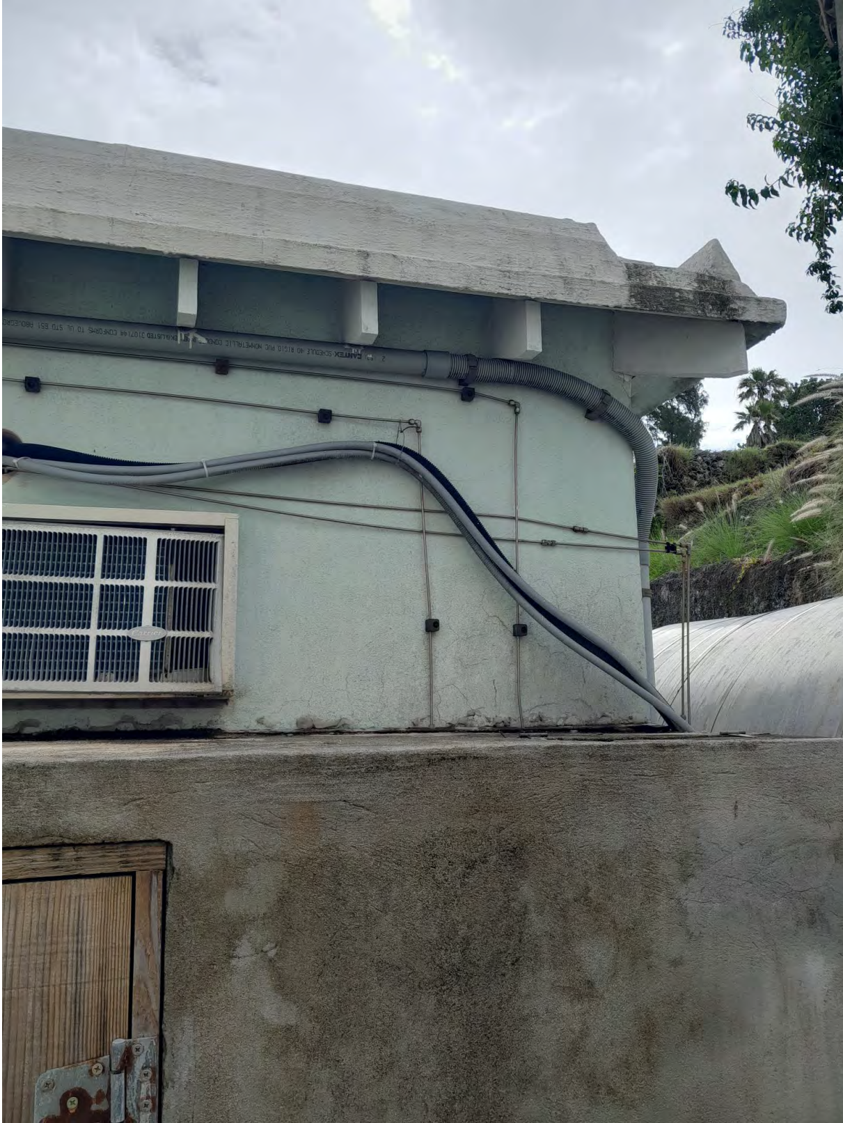
Photo 11 Gas Piping and A/C
