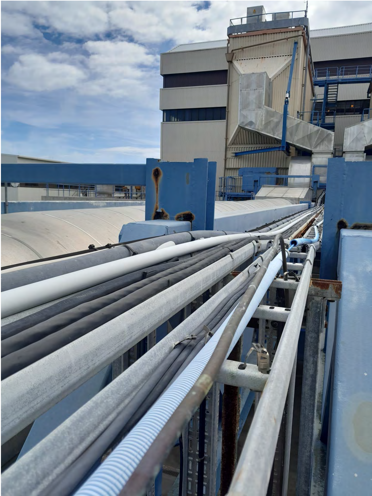
Photo 16 CEMS Wiring to Control Room
