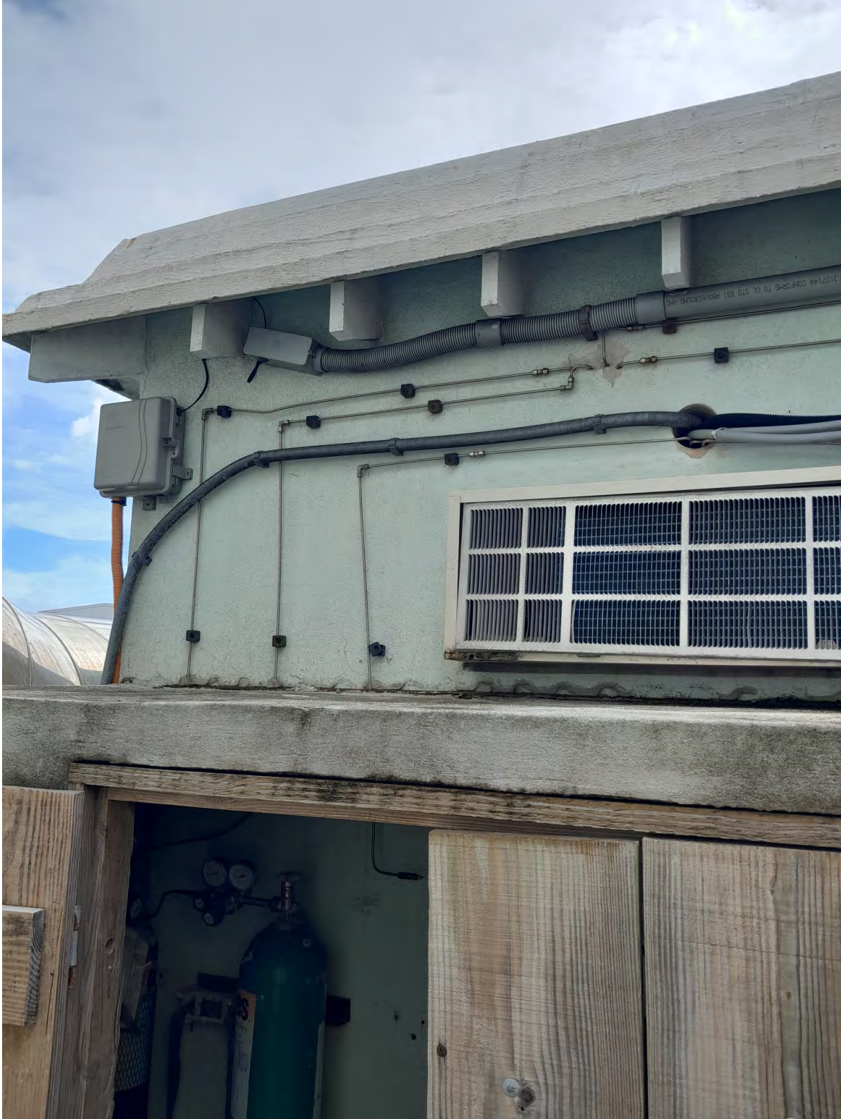
Photo 12 Gas Piping and A/C
