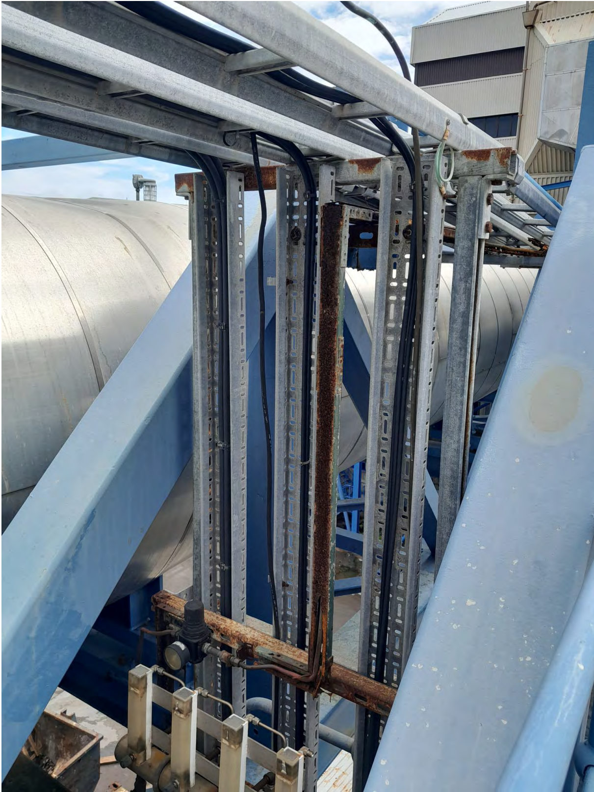
Photo 15 Typical Wiring Support
