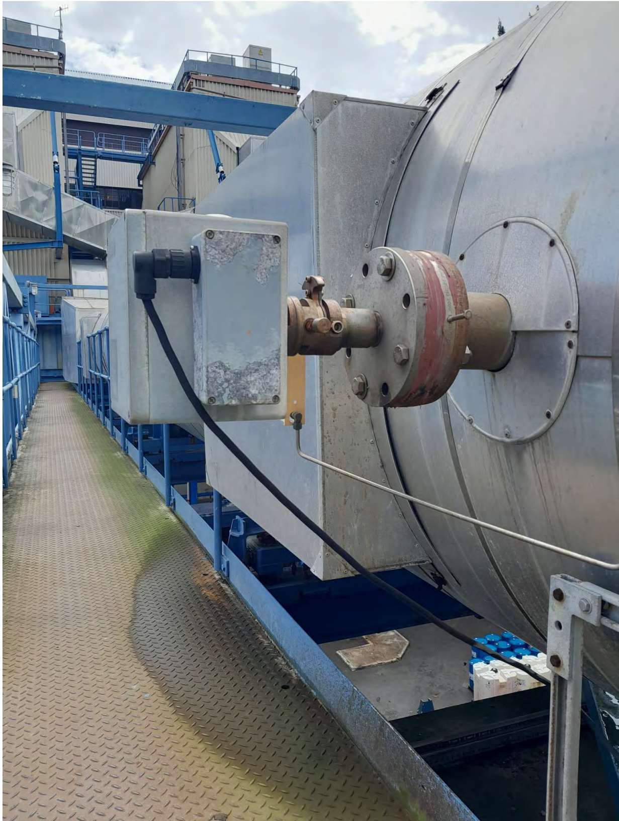
Photo 6 Typical CEMS Probe Location
