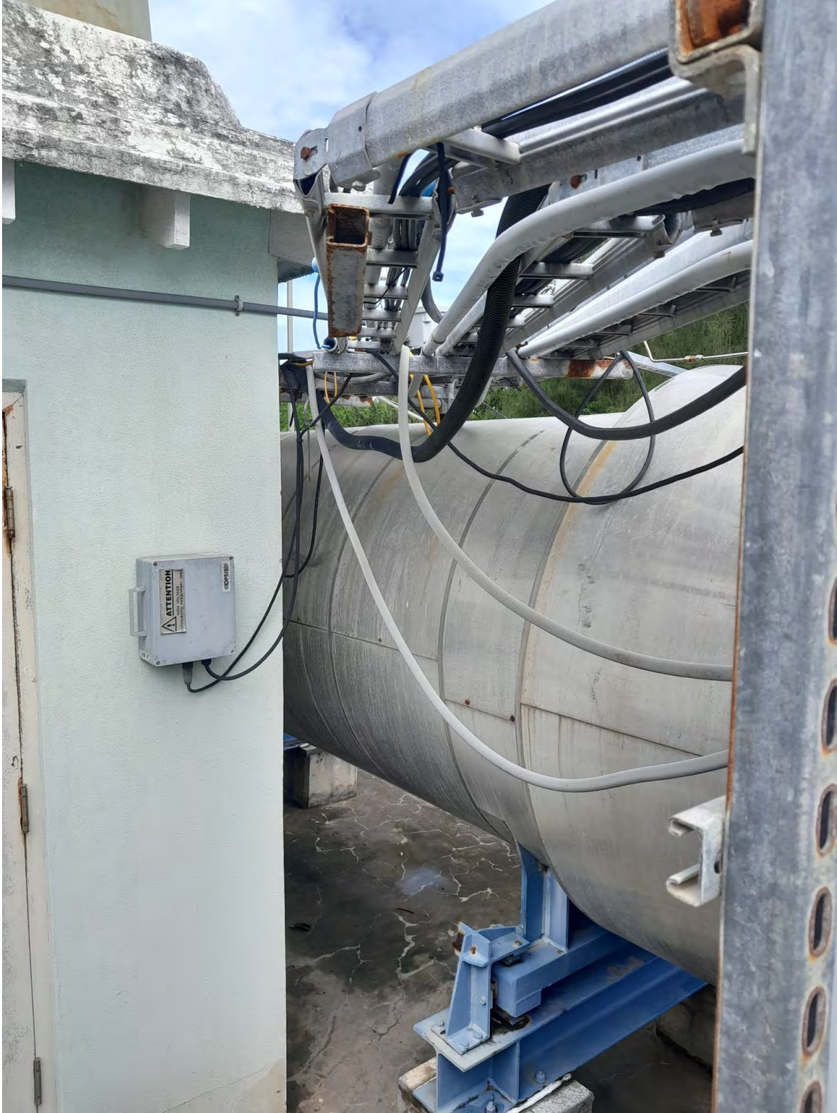
Photo 17 Typical CEMS Wiring
