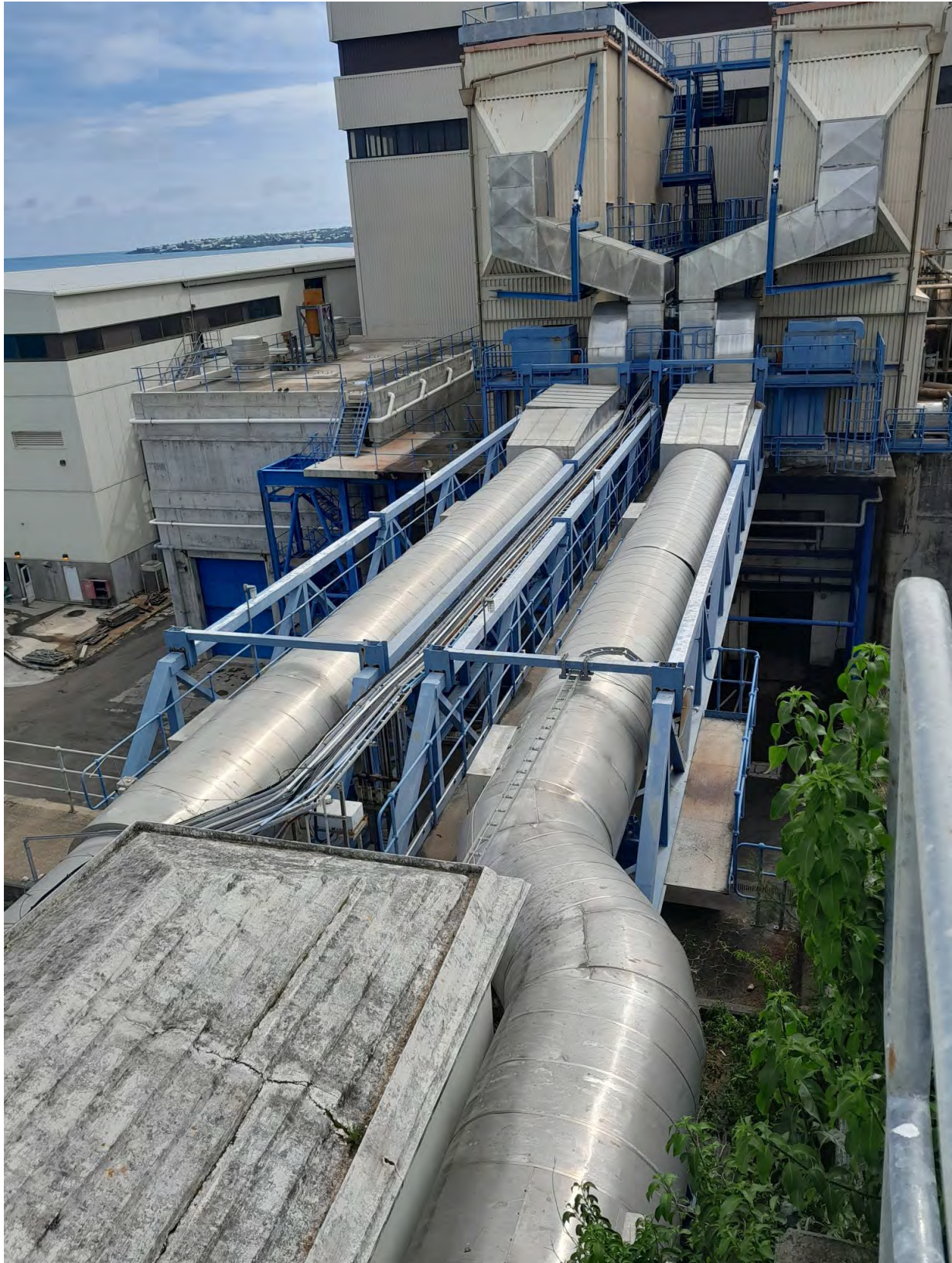
Photo 3 View of Breaching Support and Routing to Control Room
