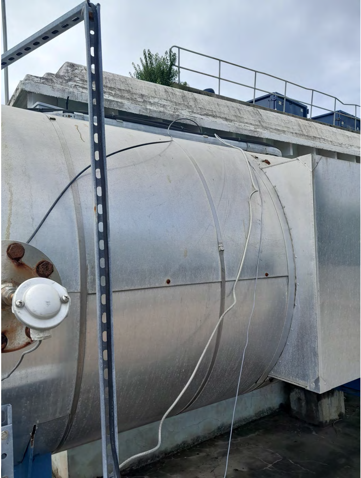
Photo 8 Existing CEMS Wiring
