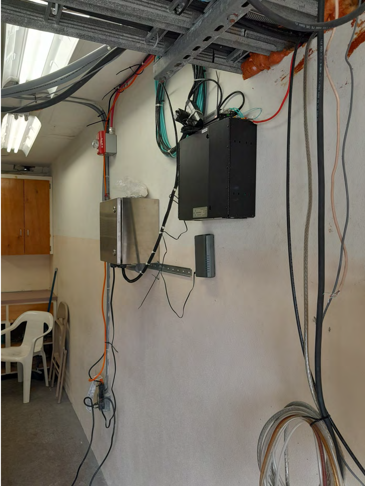
Photo 21 Typical Equipment & Wiring
