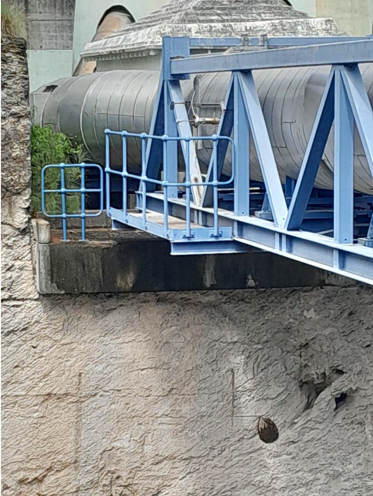
Photo 35 CEMS Equipment Access
