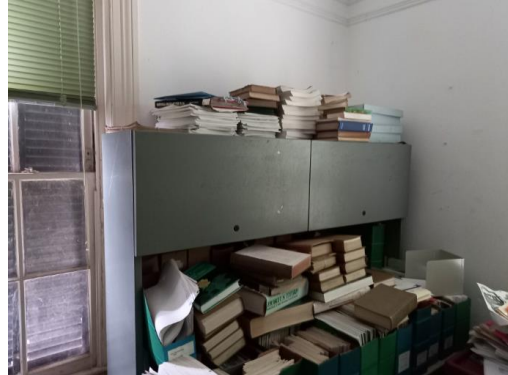
BGL- 18: Room 105, D2
