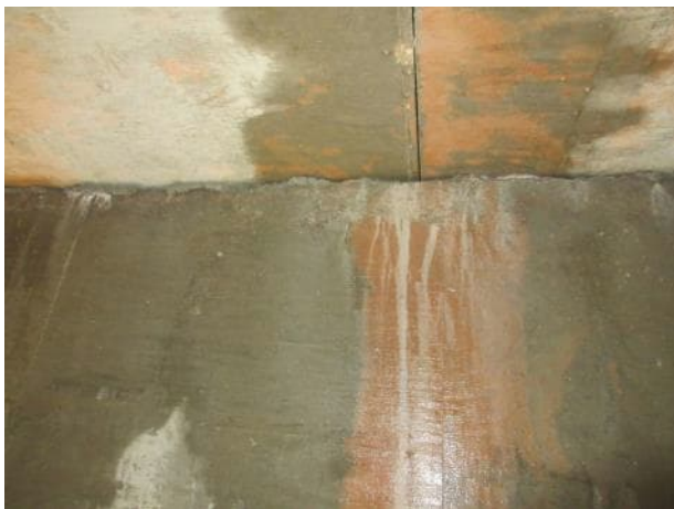
Photo 5.1.21. Water ingress over B3.
