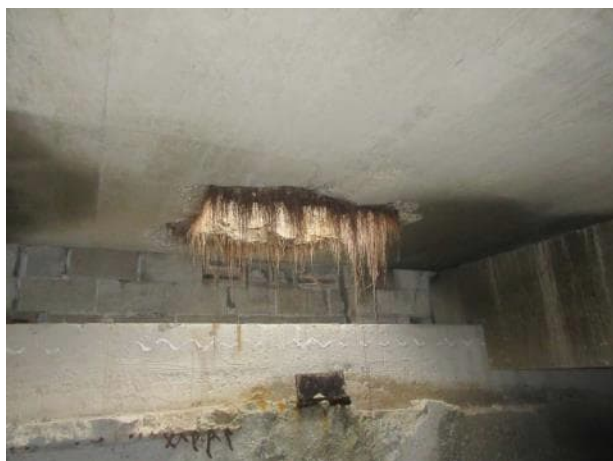
Photo 5.3.31. Roots growing in manhole.
