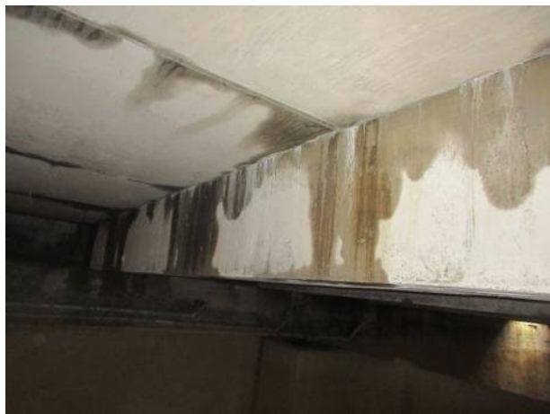
Photo 5.2.21. B9 with staining visible.
