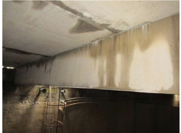
Photo 5.2.10. B7 with water ingress staining.
