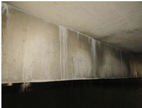
Photo 5.3.42. Beam B13 with staining visible.
