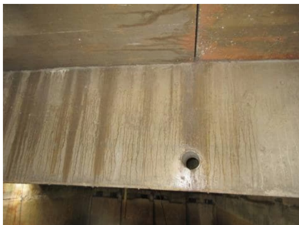
Photo 5.3.51. Beam B15 with active leaks visible.
