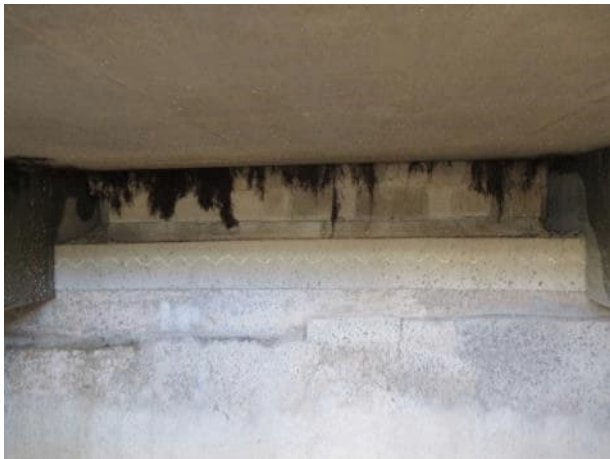
Photo 5.1.37. South bearing area between B3 and B4. Roots observed.
