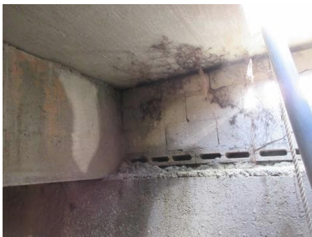
Photo 5.1.28. Beam B4 north bearing. Roots visible.
