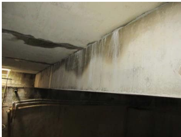
Photo 5.2.16. Beam B8 with staining visible from water ingress.
