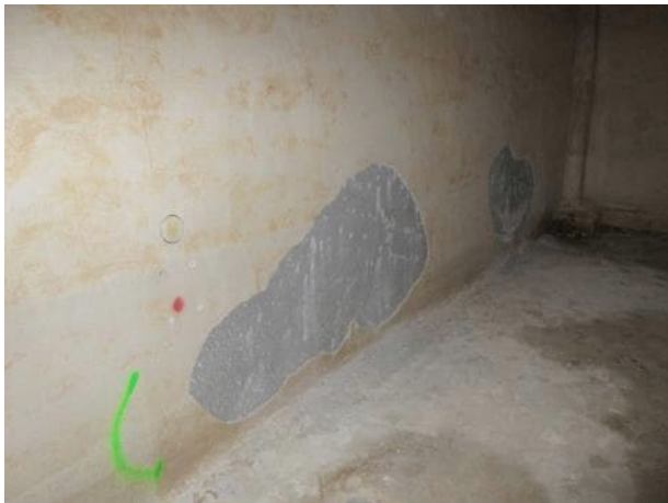
Photo 5.5.11 South wall section 2.
