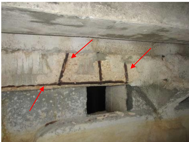
Photo 5.4.33 Corroded reinforcing was observed.
