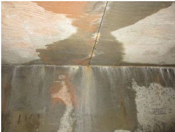
Photo 5.1.19. Typical water ingress between slabs over B2.
