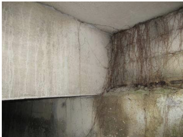
Photo 5.3.17. Beam B13 north bearing. Roots visible.
