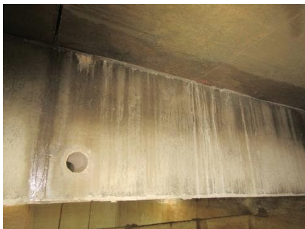
Photo 5.4.43 Staining on B17.
