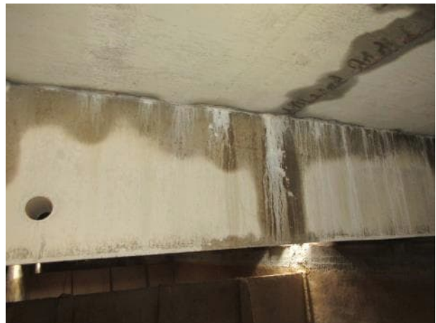
Photo 5.2.42. B8 staining and water ingress.
