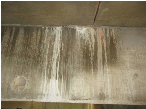
Photo 5.4.11 Staining on B17.
