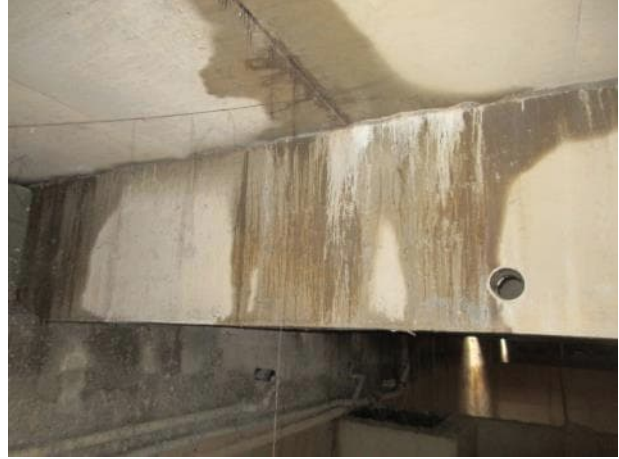
Photo 5.2.38. Deposits and staining on north side of B9.
