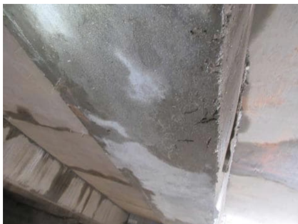
Photo 5.1.27. Old repair under B4.
