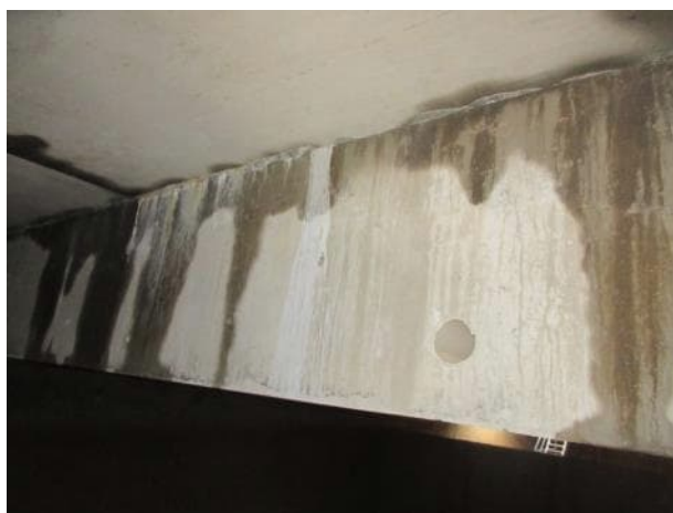
Photo 5.2.36. B9 with water staining visible.
