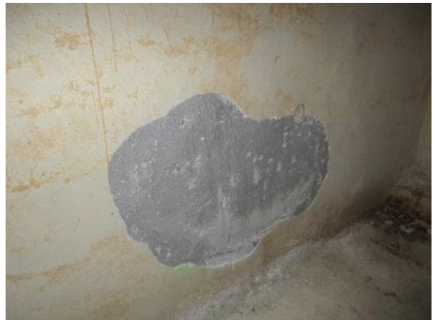
Photo 5.5.12 South wall section 2.
