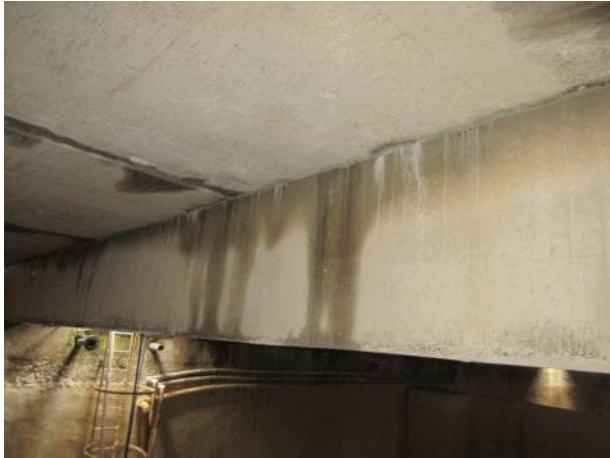
Photo 5.2.9. B7 water ingress visible.
