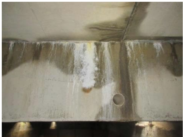
Photo 5.2.22. B9 with staining from water ingress.
