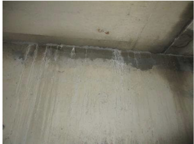
Photo 5.2.2. Water ingress and staining B6.
