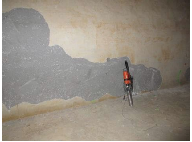
Photo 5.5.10 South wall section 2.
