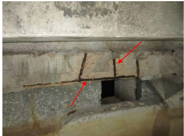
Photo 5.4.32 Corroded reinforcing steel at the eastern edge beam.
