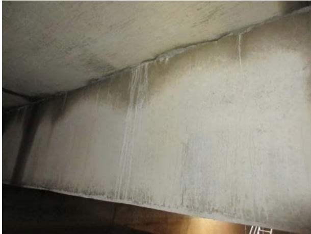
Photo 5.2.45. B7 with water staining.
