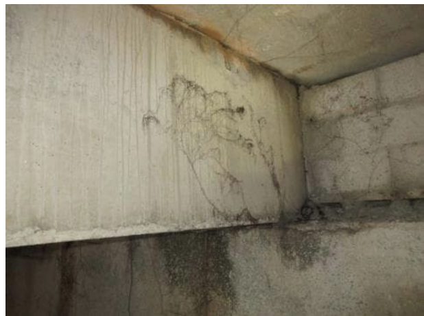
Photo 5.1.14. North bearing B2. Small roots observed.
