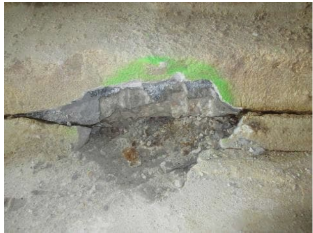
Photo 5.5.18 Exposed crack at base of wall on south side of Section 4.
