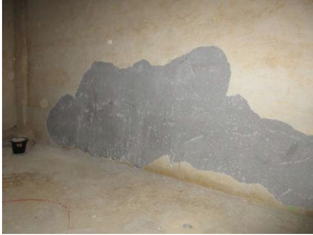
Photo 5.5.9 South wall section 2.
