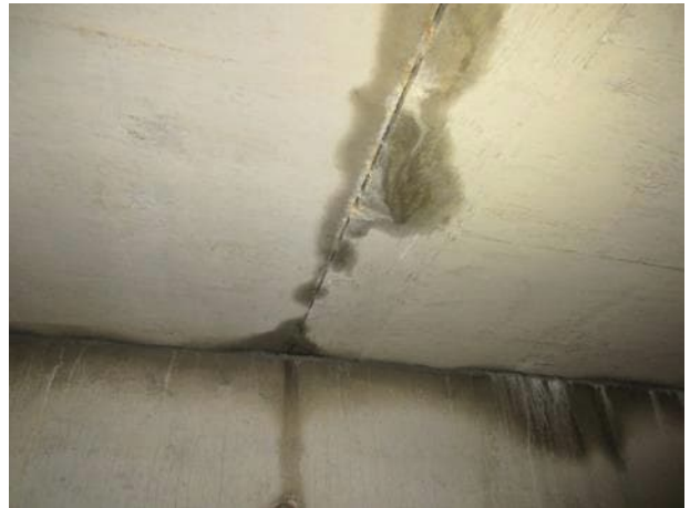
Photo 5.2.12. Water and staining visible under slab.
