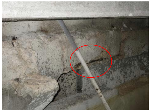
Photo 5.4.34 Corroded reinforcing at eastern edge beam.
