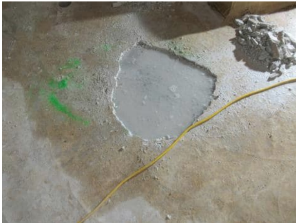
Photo 5.5.1 Hollow section in Section 3 Floor (eastern end).
