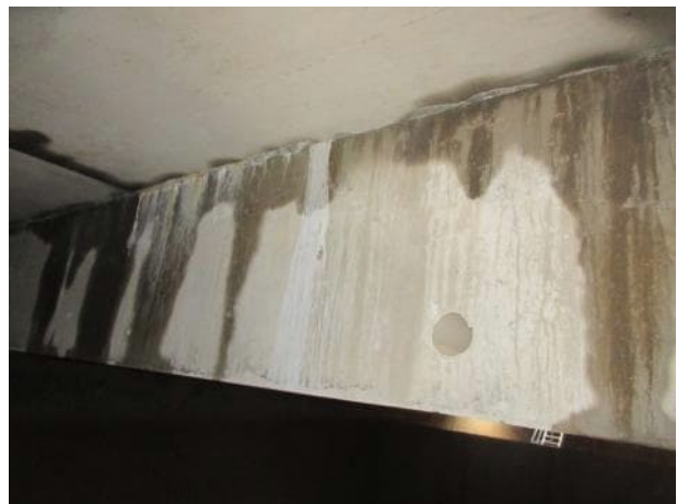
Photo 5.2.36. B9 with water staining visible.
