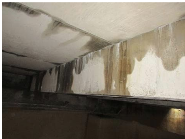
Photo 5.2.21. B9 with staining visible.
