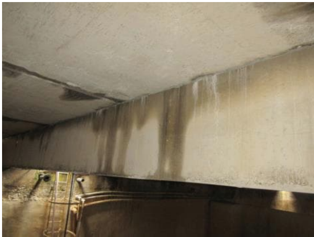
Photo 5.2.9. B7 water ingress visible.
