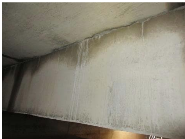
Photo 5.2.45. B7 with water staining.
