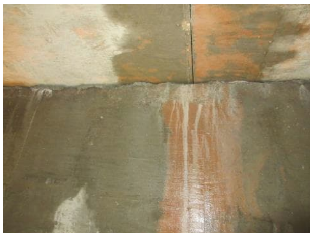
Photo 5.1.21. Water ingress over B3.
