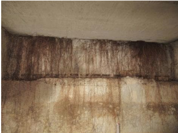
Photo 5.3.1. North bearing between B11 and B12. Roots observed.
