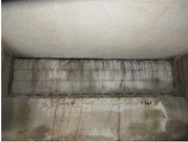
Photo 5.3.23. North bearing area between B14 and B15. Tree roots observed.
