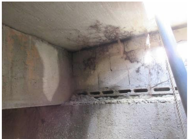
Photo 5.1.28. Beam B4 north bearing. Roots visible.
