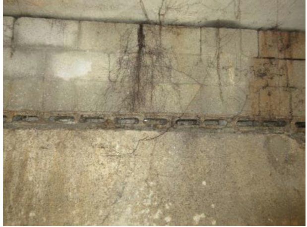
Photo 5.1.24. North Bearing area between B3 and B4. Roots observed growing into concrete block.
