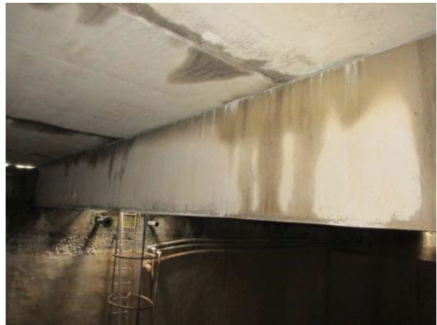
Photo 5.2.10. B7 with water ingress staining.
