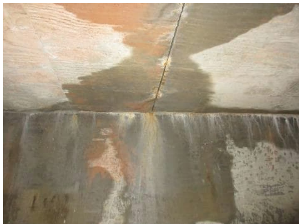
Photo 5.1.19. Typical water ingress between slabs over B2.
