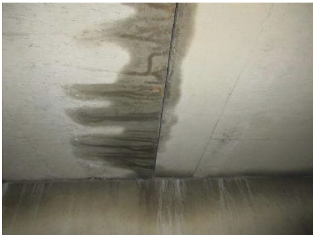
Photo 5.2.5. Water ingress between slabs.
