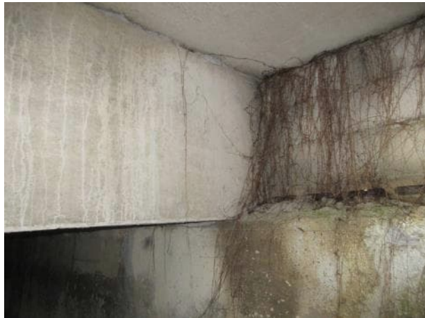
Photo 5.3.17. Beam B13 north bearing. Roots visible.
