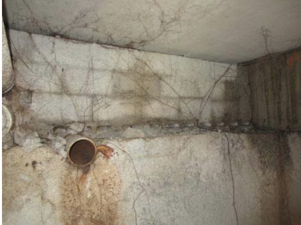
Photo 5.1.1. North bearing between B1 and B2. Roots visible.
