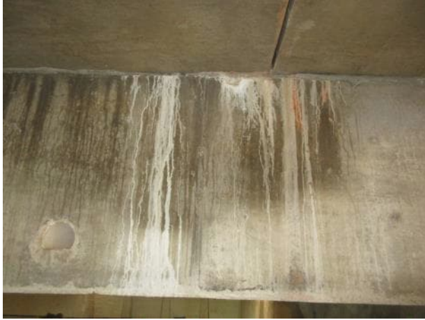
Photo 5.4.11 Staining on B17.
