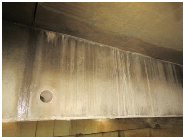
Photo 5.4.43 Staining on B17.
