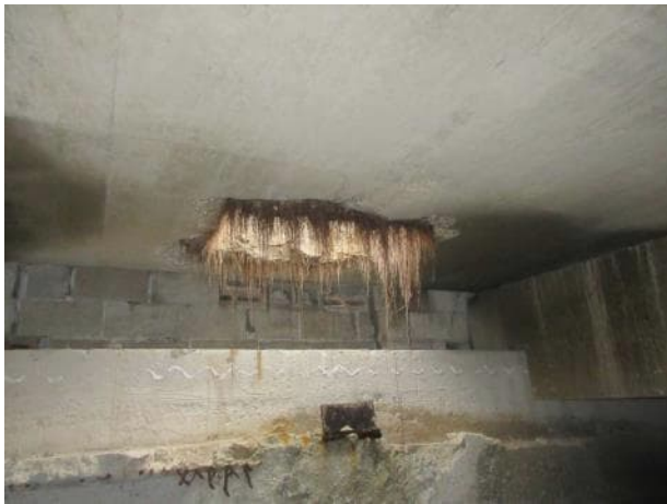
Photo 5.3.31. Roots growing in manhole.
