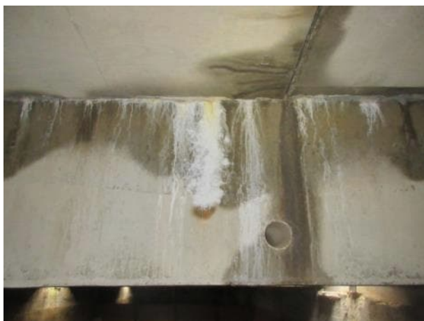
Photo 5.2.22. B9 with staining from water ingress.
