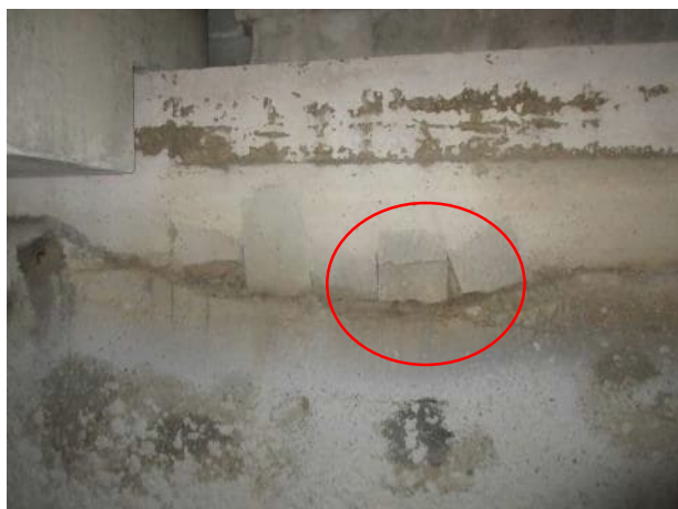
Photo 5.3.45. Minor damage to concrete block between B13 and B14.
