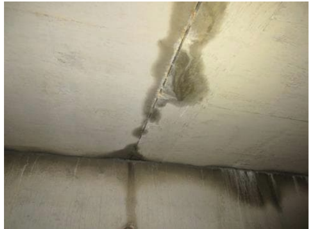
Photo 5.2.12. Water and staining visible under slab.
