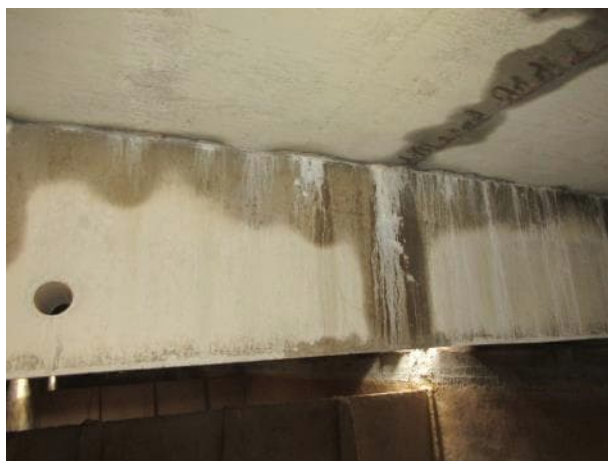
Photo 5.2.42. B8 staining and water ingress.
