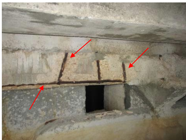
Photo 5.4.33 Corroded reinforcing was observed.
