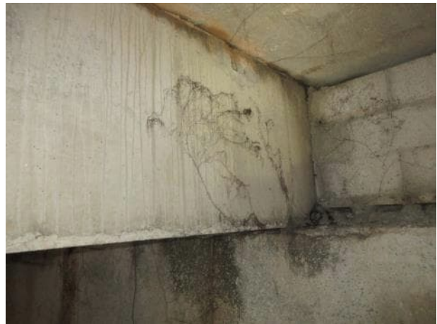
Photo 5.1.14. North bearing B2. Small roots observed.
