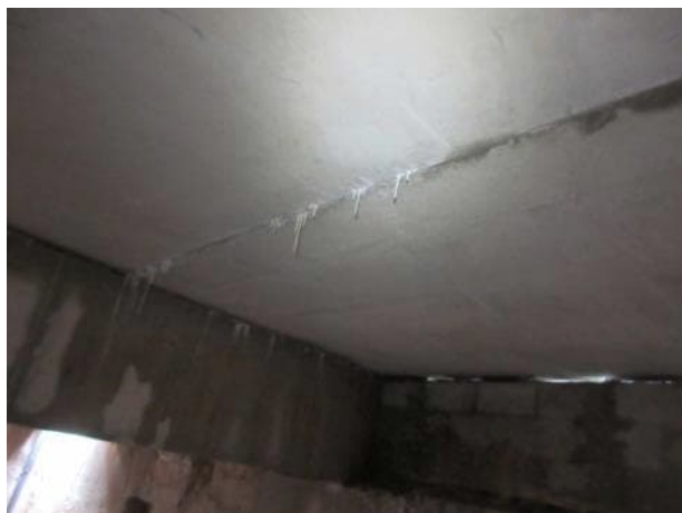
Photo 5.2.47. Deposits from water ingress between B5 and B6.
