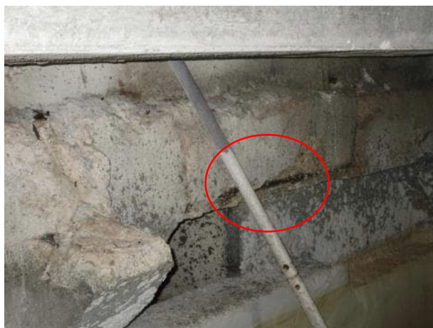
Photo 5.4.34 Corroded reinforcing at eastern edge beam.
