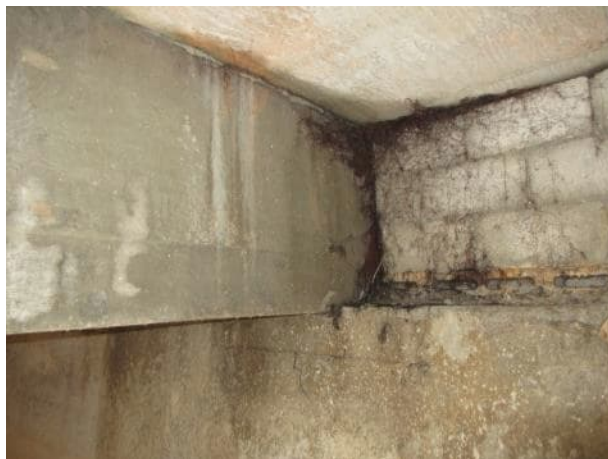
Photo 5.1.20. North bearing of B3. Roots visible.
